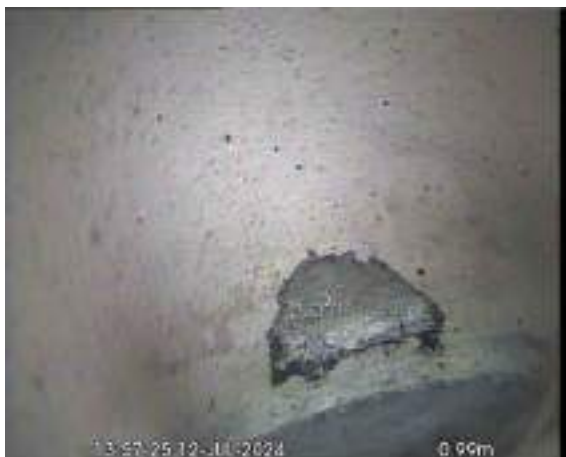
GULLYX_6d63e6bc-a192-46ee-bb28-5b54a1a3e0d8_20240725_095748_794.jpg, 00:00:39, 0.99 m Finish node, gully, reference: GULLY
