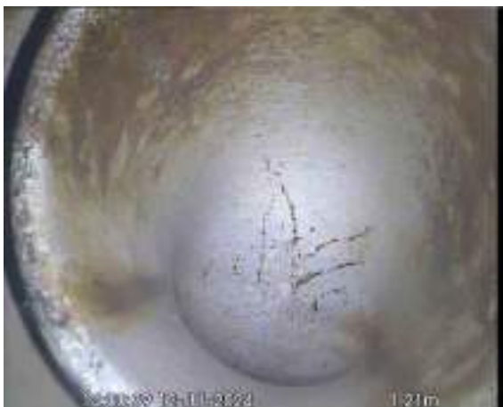
GULLYX_0146e961-7b26-494e-83c0-d047bf27c81e_20240725_101142_978.jpg, 00:00:31, 1.21 m Finish node, gully, reference: GULLY
