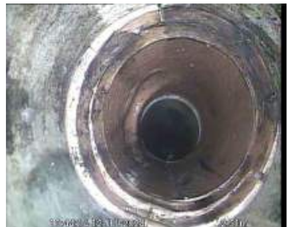
MH6X_5b7b7237-2ba3-4cba-86aa-fcb1f22d1ecc_20240725_092232_813.jpg, 00:00:41, 2.51 m Fracture, multiple at joint from 12 o'clock to 12 o'clock
