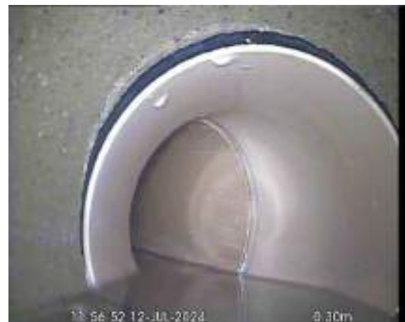
MH2X_9e3848a9-2aef-4403-9dc0-06a55e9cccf0_20240725_092609_653.jpg, 00:00:56, 0.30 m Joint displaced, medium
