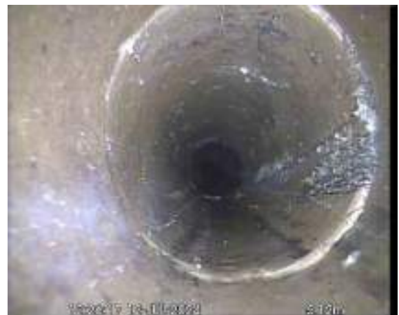
MH5X_109efa46-164d-464f-96dd-18bcad47188e_20240725_094816_811.jpg, 00:01:44, 5.12 m Roots, fine at joint
