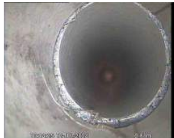
GULLYX_497c7feb-53ee-44b1-89dc-872bd2b7a9cf_20240725_090218_006.jpg, 00:01:01, 0.81 m Roots, fine at joint
