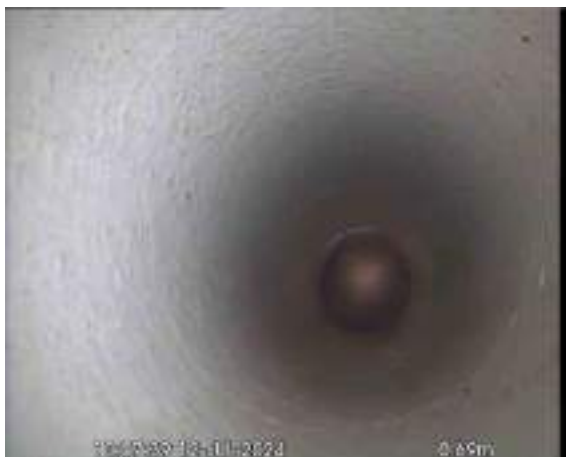
W_CX_6de99cdf-b413-404c-b955-bd55d3022d42_20240725_090601_206.jpg, 00:00:31, 0.69 m Crack, circumferential from 3 o'clock to 8 o'clock
