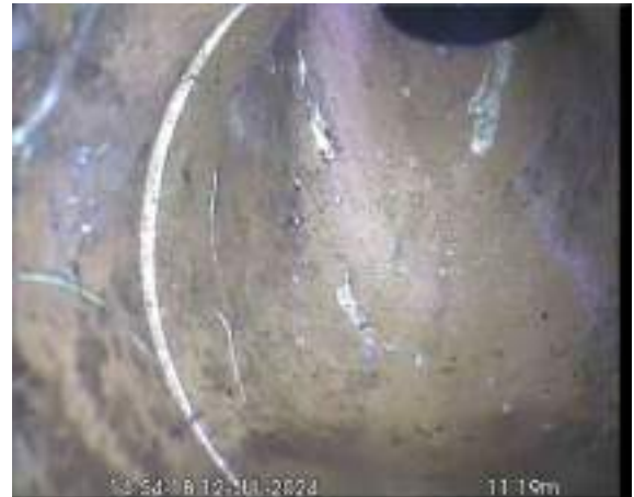
RWDPX_86dc6ebb-da85-45a0-a40c-1b8118d31bb7_20240725_101744_768.jpg, 00:01:49, 11.19 m Line deviates up, REST BEND
