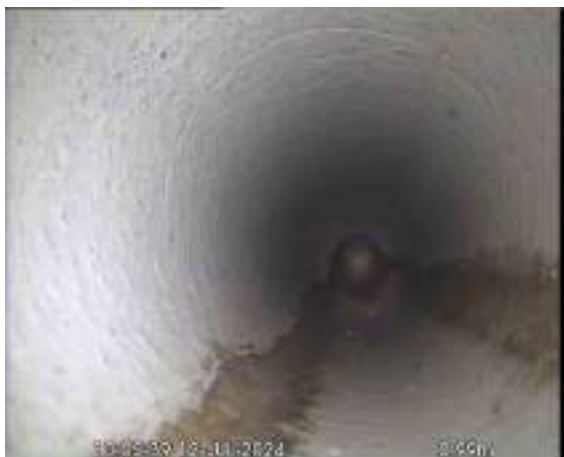
W_CX_b0b5a396-c87b-44df-b524-f6ae86763abc_20240725_090413_863.jpg, 00:00:37, 0.99 m Crack, circumferential from 9 o'clock to 3 o'clock
