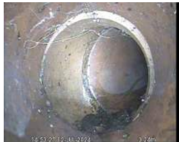
RWDPX_b04b44a7-7c3f-4146-a3f3-0906ec81aae0_20240725_101714_425.jpg, 00:00:58, 3.24 m Line deviates right
