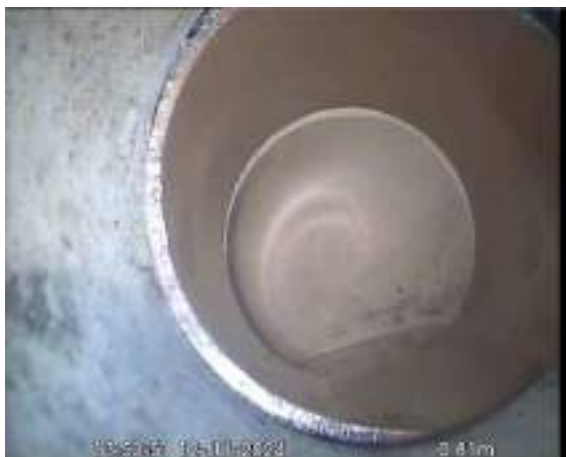
SVPX_6126ff3a-8feb-42cf-b4a8-289a35627abd_20240725_095243_344.jpg, 00:00:43, 0.81 m Joint displaced, medium
