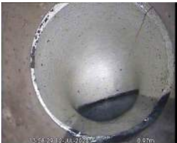
GULLYX_36dc49d5-3dc1-4da4-862e-24eaa0b586df_20240725_100014_047.jpg, 00:00:24, 0.97 m Crack, longitudinal at joint at 2 o'clock
