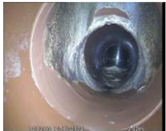
GULLYX_299e09be-81f4-44b5-a1cc-c1a653637af6_20240725_101416_847.jpg, 00:01:16, 3.42 m Junction at 12 o'clock, diameter: 110mm, W/C
