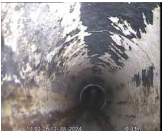
GULLYX_2b29d929-3dfa-4401-bebe-b29732e2f259_20240725_101316_226.jpg, 00:00:39, 0.43 m Fracture, circumferential from 10 o'clock to 3 o'clock
