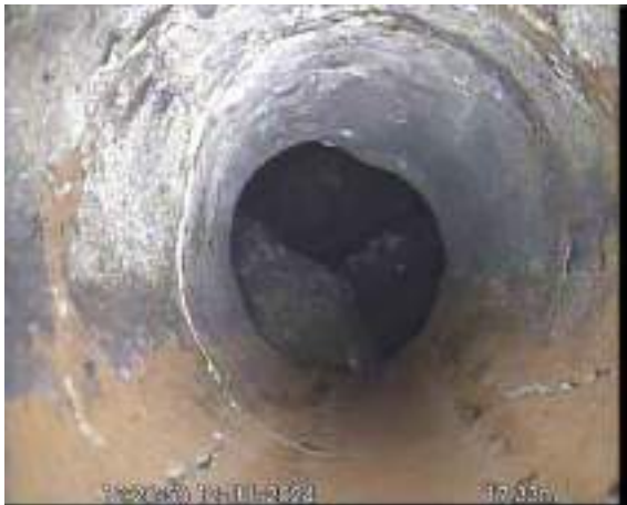
MH5X_245e56e0-af60-4cc5-9251-72fe8d11e2b2_20240725_094946_179.jpg, 00:02:23, 17.33 m Fracture, multiple from 12 o'clock to 12 o'clock
