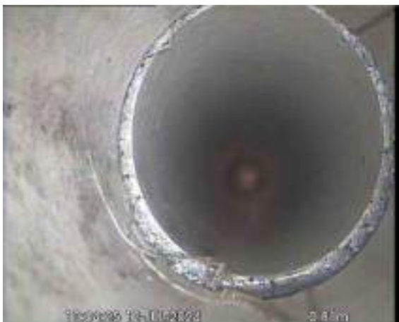
GULLYX_b10122b8-1f1f-4b61-85ad-1d1dd839dd63_20240725_090208_797.jpg, 00:01:01, 0.81 m Crack, circumferential at joint from 6 o'clock to 9 o'clock
