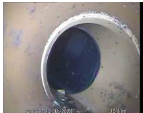
MH4X_9d8f4504-f323-432b-9698-14d451cd618f_20240725_094016_482.jpg, 00:01:29, 15.81 m Line deviates left
