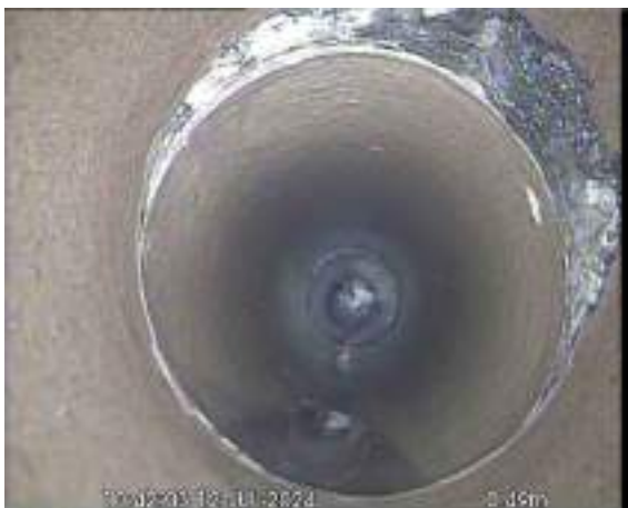
REDUNDANTX_0df9520d-4cc8-45ca-b8b9-6ea8c8cc1138_20 240725_091130_965.jpg, 00:00:34, 0.49 m Joint displaced, large
