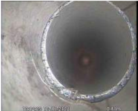
GULLYX_be408751-b267-4dcb-87b2-47920da53df0_20240725_090226_317.jpg, 00:01:01, 0.81 m Joint displaced, medium
