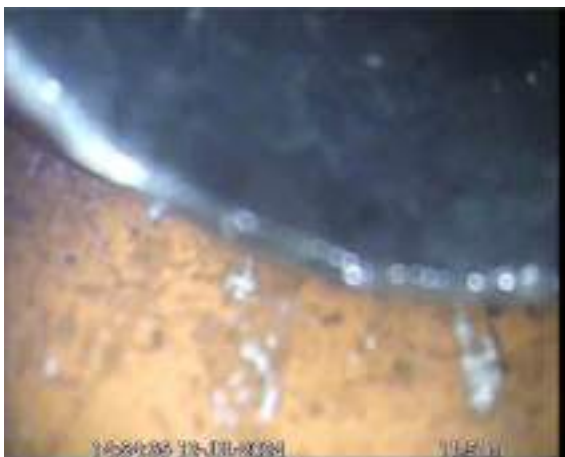
RWDPX_f74d9b74-efa2-4767-b22b-1b8d34b363b9_20240725_101807_038.jpg, 00:02:06, 11.51 m Finish node, major connection without manhole, reference: RAINWATER DOWNPIPE (RWDP)
