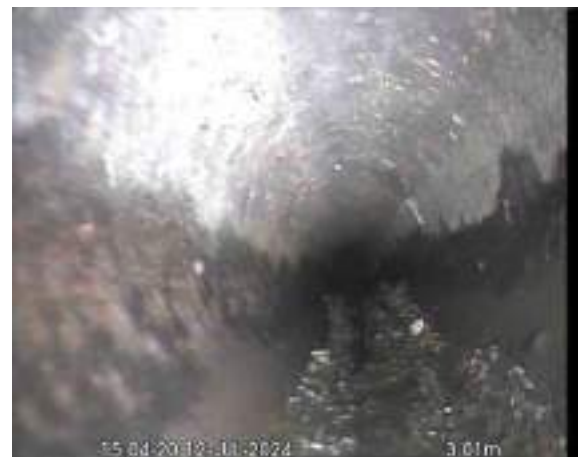
MANHOLEX_9f739453-0b6d-4c3b-aa2f-970cef82bb99_20240725_102213_871.jpg, 00:00:51, 3.01 m Settled deposits, fine, 5% cross-sectional area loss
