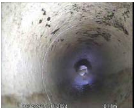
MH1X_97e7b7b8-20ed-4a65-9726-8e0e94167fbc_20240725_090948_059.jpg, 00:00:28, 0.18 m Crack, circumferential from 6 o'clock to 12 o'clock
