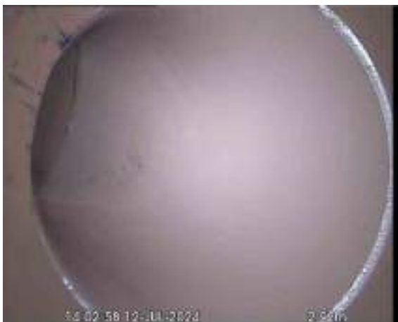
GULLYX_0fb9ef59-34cb-4c01-8650-9407a85952f5_20240725_101359_633.jpg, 00:01:09, 2.92 m Line deviates left
