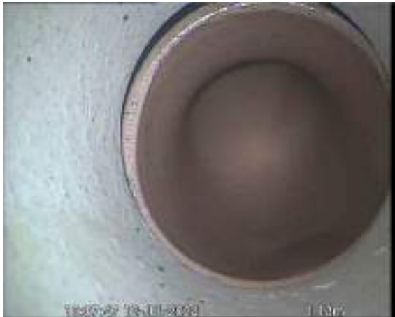
W_CX_1865770f-a7a0-438a-95c3-9da68d53db4d_20240725_090701_492.jpg, 00:00:39, 1.13 m Joint displaced, medium
