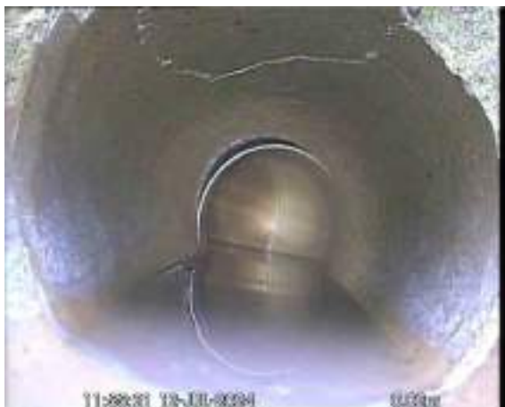
MH2X_71538d31-1645-4ac7-b3ba-3a632e838191_20240725_092525_584.jpg, 00:00:35, 0.02 m Crack, circumferential from 10 o'clock to 2 o'clock
