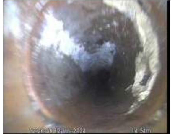
MH5X_b9529b71-08d6-4df3-a0ef-83327201d51f_20240725_094926_931.jpg, 00:02:15, 14.54 m Hole in drain or sewer at 4 o'clock
