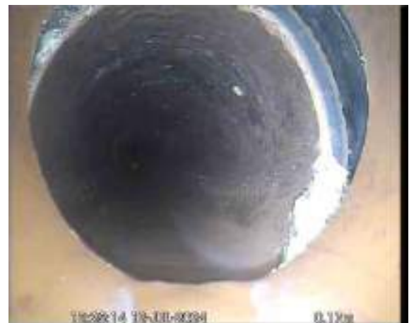
MH5X_f2943572-daea-4cc0-b643-02d9ae5cd5ee_20240725_094641_129.jpg, 00:00:44, 0.17 m Material changes to vitrified clay
