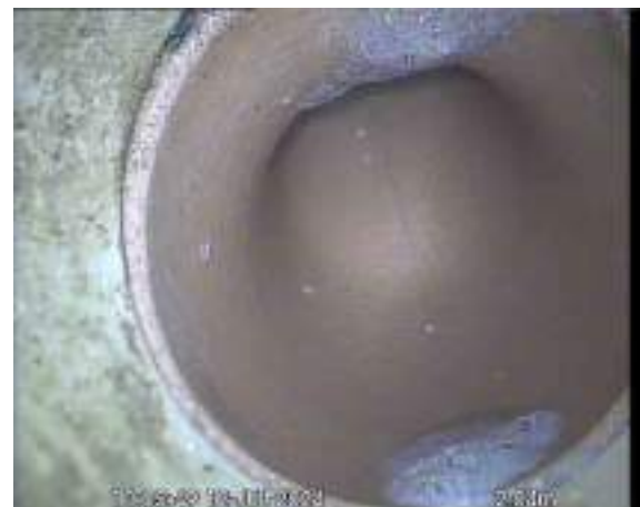
W_CX_96eda4f4-1bbb-49c3-bdf5-b6f3418d49e6_20240725_090429_528.jpg, 00:00:47, 2.04 m Line deviates up, REST BEND
