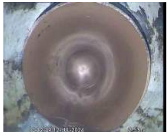
GULLYX_a0d2ed5e-7b7e-4ae5-a077-94c7952a4929_20240725_101329_585.jpg, 00:01:00, 2.53 m Joint displaced, medium
