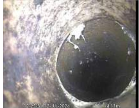
MH5X_059f6707-2778-4d9f-998a-3e91e87c5d40_20240725_094727_709.jpg, 00:01:24, 4.11 m Joint displaced, medium
