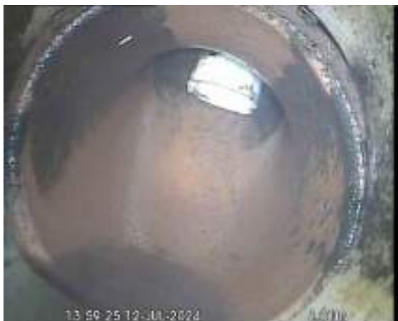
BASINX_40e5934f-6751-4c2f-8103-7d817af70ed0_20240725_101004_289.jpg, 00:00:28, 1.01 m Line deviates up, REST BEND
