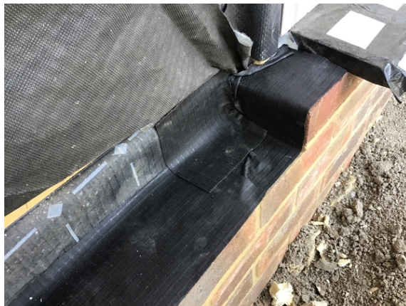
External door threshold detailing to plot 34.
