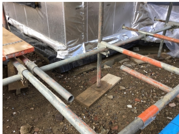
Evidence of the outer brickwork not in place to all plots noted above at the time of our inspection.
