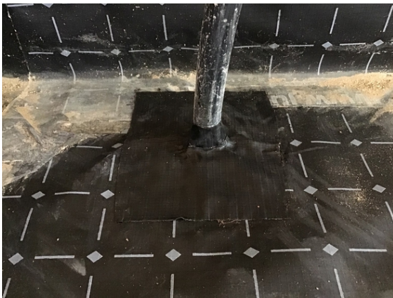
Pipe penetration detailing in plot 26.
