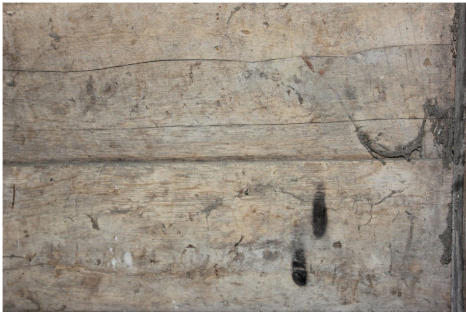
Plate 36. Taper burns marks on the south side of the threshing partition.
