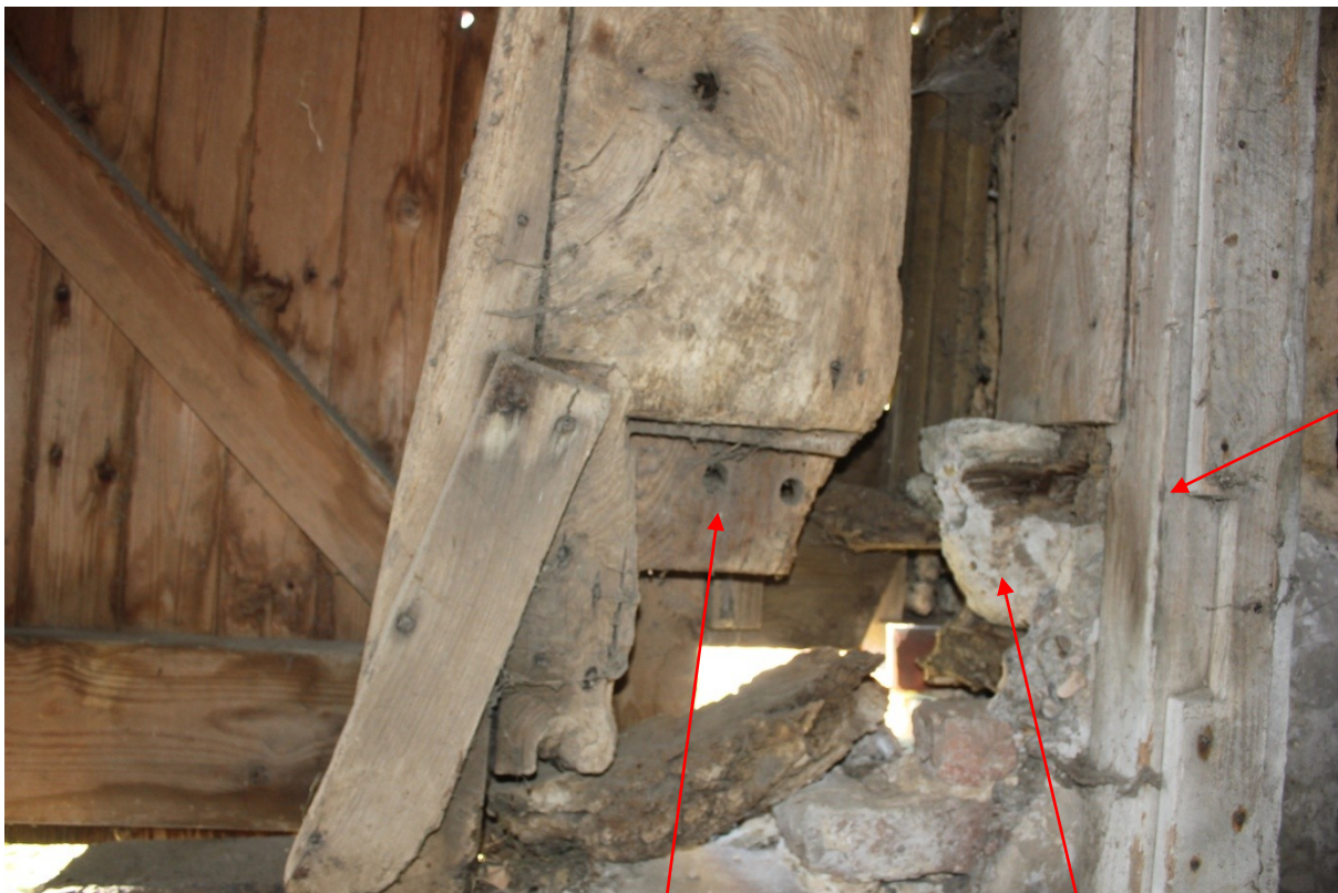
Plate 19. Substantial posts of the internal frame were tenoned to the cill beam (now rotted).
