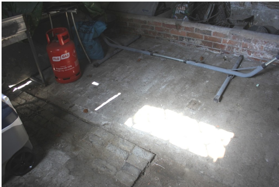
Plate 29. The brick flooring in the outshot covered by cementitious slurry.
