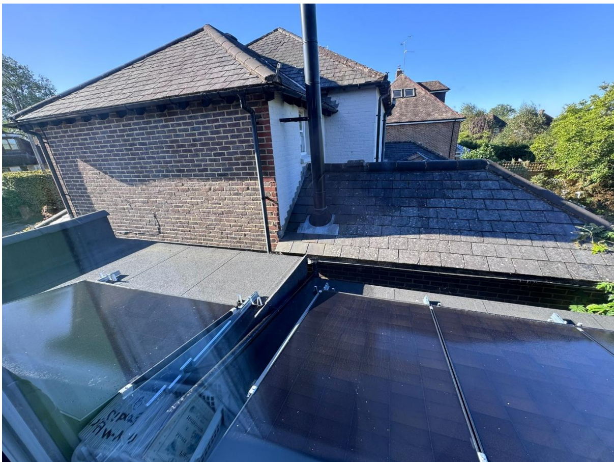
Figure 10: Solar panels and Hamsey Cottage, including its oil boiler flue
