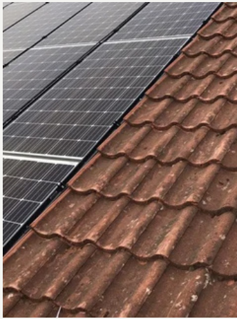
INTEGRATED SOLAR PANELS
