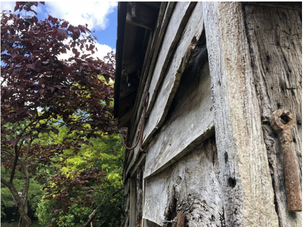
Photograph 2. Gaps between weather boarding on the western elevation of the annexe.
