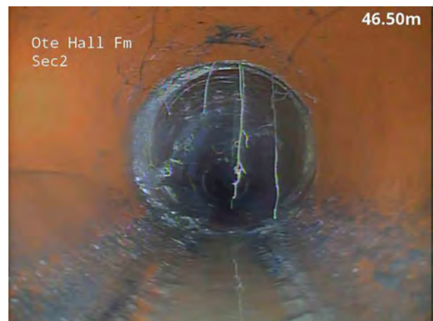
16, 00:02:21, 46.70 m Roots, fine at joint
