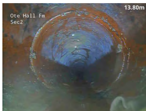
10, 00:05:23, 14.00 m Fracture, circumferential at joint from 12 o'clock to 12 o'clock
