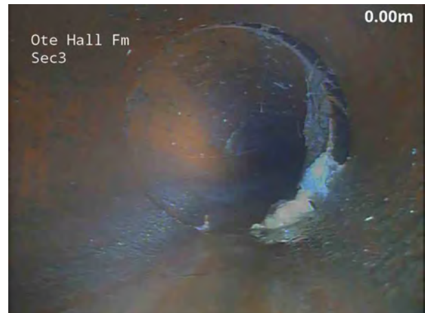
2, 00:00:11, 0.30 m Roots, fine at joint
