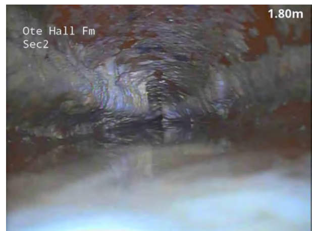
6, 00:00:29, 2.00 m Attached deposits, grease from 9 o'clock to 3 o'clock, 25% cross-sectional area loss, change
