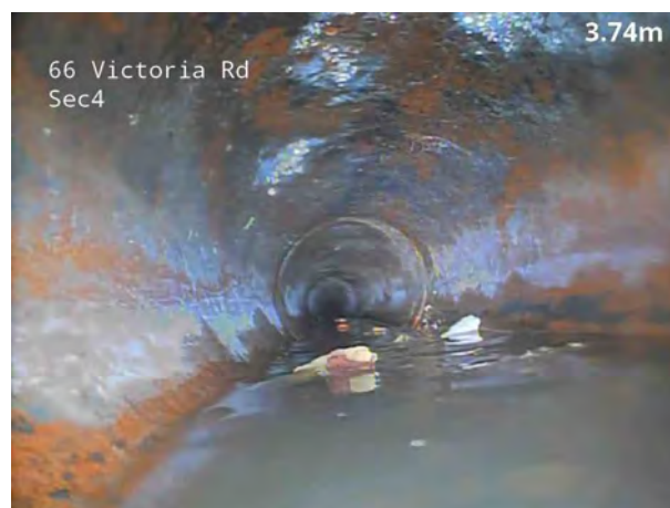
6, 00:00:30, 3.80 m Settled deposits, coarse, 15% cross-sectional area loss, change
