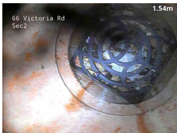
3, 00:00:29, 1.60 m Finish node, manhole, reference: GY
