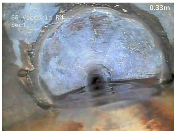
3, 00:00:22, 0.50 m Fracture, circumferential at joint from 8 o'clock to 5 o'clock
