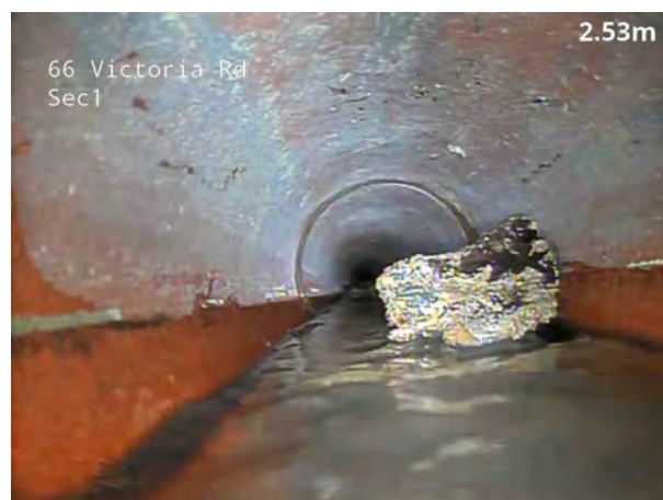
6, 00:00:51, 2.50 m Attached deposits, other from 4 o'clock to 8 o'clock, 15% cross-sectional area loss, start
