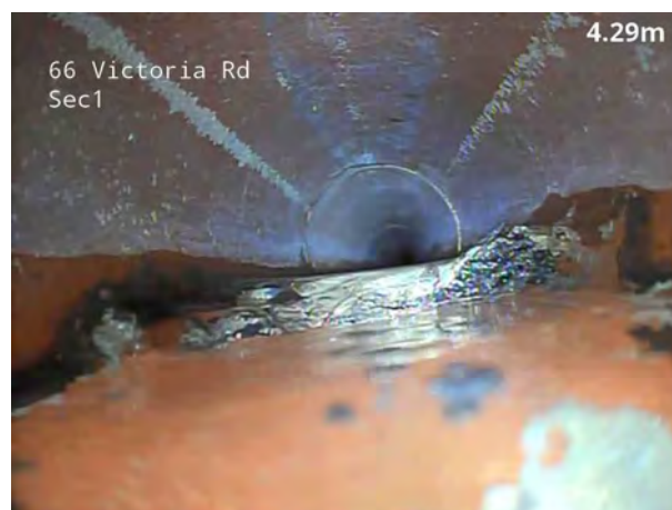
8, 00:01:06, 4.40 m Attached deposits, other from 3 o'clock to 9 o'clock, 20% cross-sectional area loss, change
