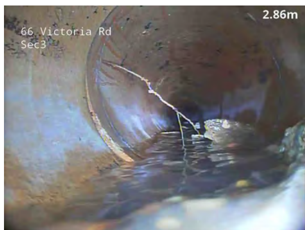
3, 00:00:30, 3.10 m Settled deposits, coarse, 10% cross-sectional area loss
