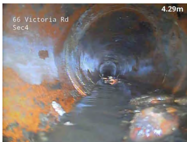
7, 00:00:44, 4.50 m Fracture, circumferential at joint from 12 o'clock to 12 o'clock
