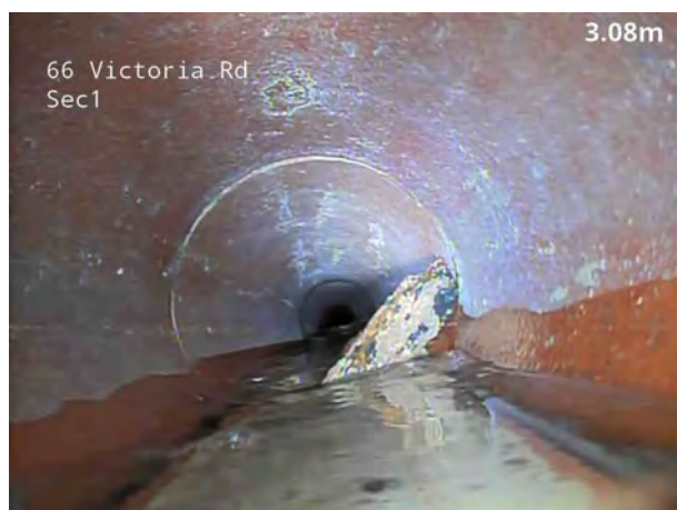
7, 00:00:57, 3.30 m Settled deposits, coarse, 20% cross-sectional area loss
