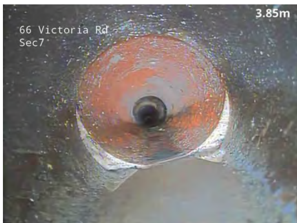
5, 00:00:38, 4.00 m Joint displaced, medium
