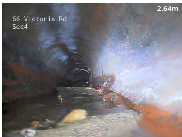
5, 00:00:24, 2.70 m Settled deposits, coarse, 20% cross-sectional area loss, change
