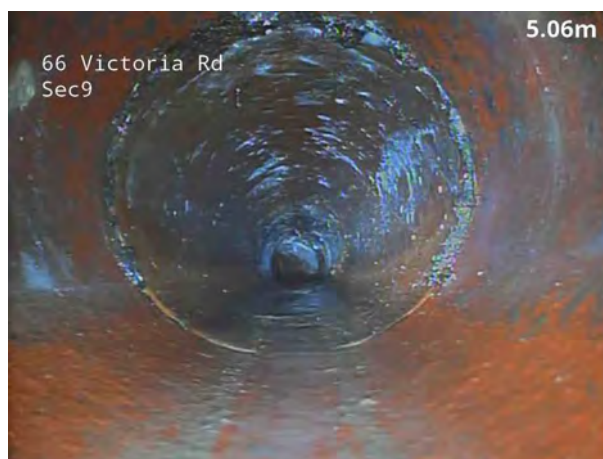
2, 00:00:45, 5.20 m Roots, fine at joint
