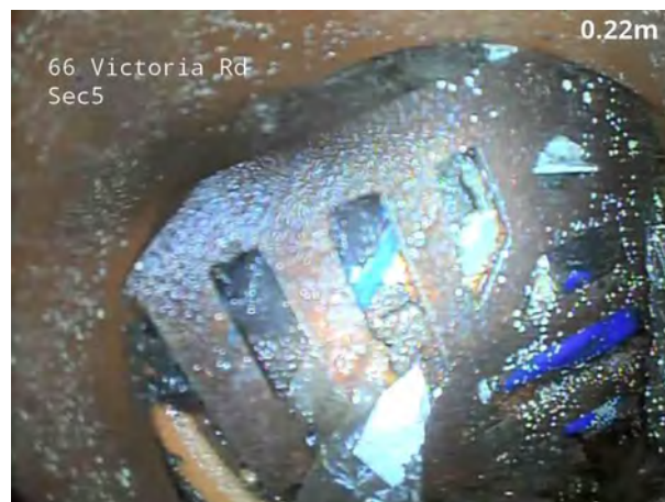
2, 00:00:12, 0.40 m Settled deposits, coarse, 100% cross-sectional area loss, Broken gully grill
