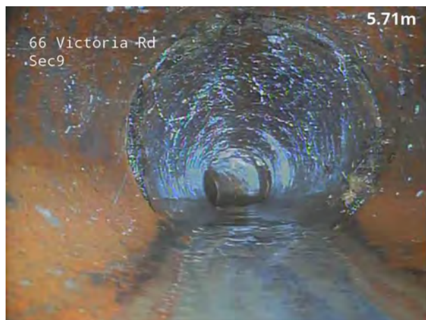
3, 00:00:48, 6.00 m Roots, fine at joint
