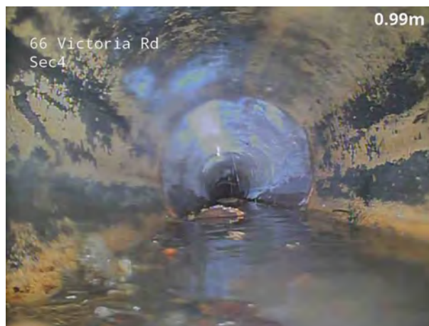
4, 00:00:13, 1.00 m Settled deposits, coarse, 15% cross-sectional area loss, change
