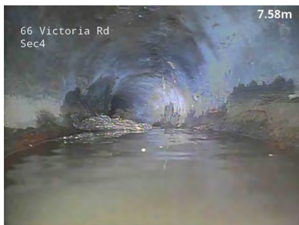
11, 00:01:05, 7.80 m Settled deposits, coarse, 10% cross-sectional area loss
