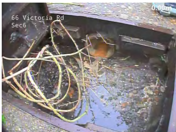
1, 00:00:00, 0.00 m Start node, manhole, reference: ACO
