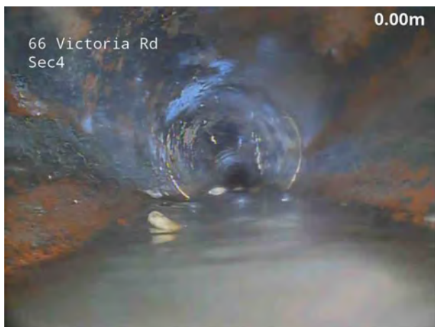
3, 00:00:06, 0.00 m Settled deposits, coarse, 10% cross-sectional area loss, start
