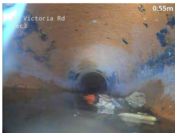
2, 00:00:19, 0.70 m Settled deposits, coarse, 15% cross-sectional area loss, start
