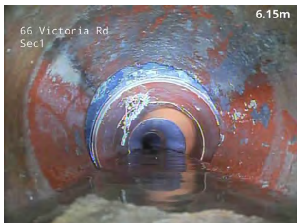
9, 00:01:19, 6.40 m Attached deposits, other from 3 o'clock to 9 o'clock, 20% cross-sectional area loss, finish
