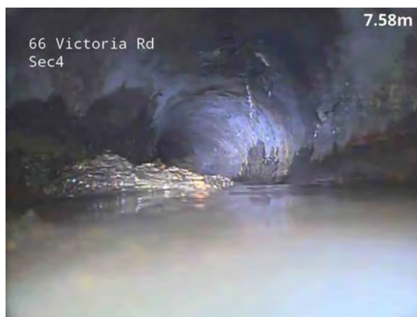
10, 00:01:02, 7.80 m Other obstacles from 4 o'clock to 9 o'clock, 30% cross-sectional area loss
