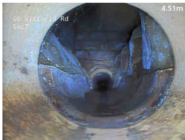
6, 00:00:45, 4.70 m Finish node, manhole, reference: FW2, Internal
