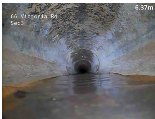
4, 00:00:42, 6.40 m Settled deposits, coarse, 5% cross-sectional area loss, change
