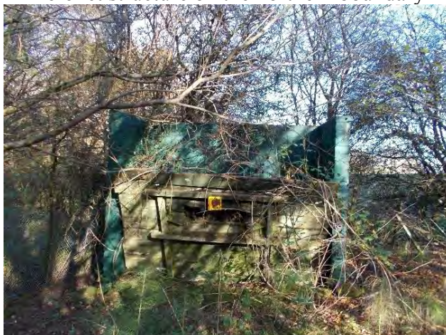
Derelict structure on the northern boundary
