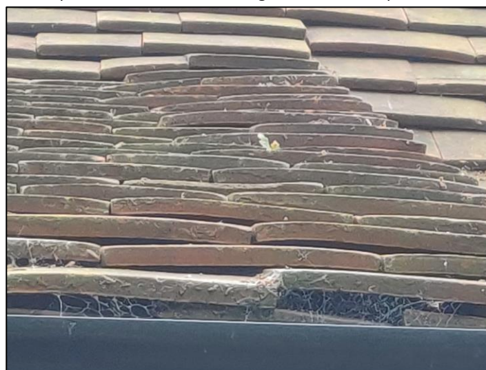
Photo 4.4: Gaps beneath lifted tiles along the northern aspect of building B1a.
