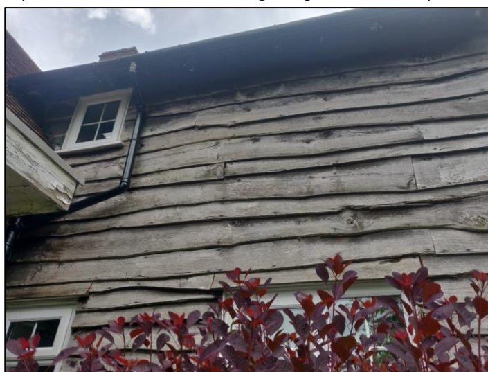
Photo 4.5: Gaps beneath the wooden cladding along the western aspect of building B1a.
