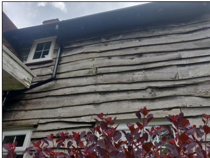
Photo 4.3: Gaps beneath the wooden cladding along the western aspect of building B1a.
