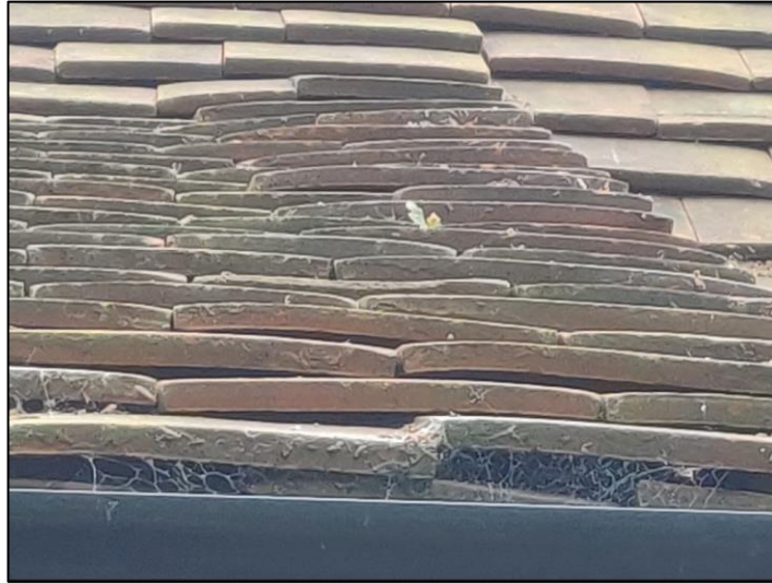
Photo 4.2: Gaps beneath lifted tiles along the northern aspect of building B1a.
