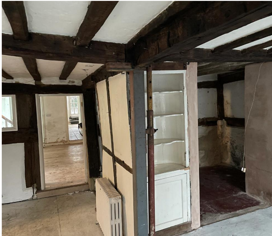
Figure 14: Central supporting post to main living room. The partitions to the small snug room were of largely modern construction. Source: McCarey Simmonds, Structural Inspection Report of 15 th March 2023
