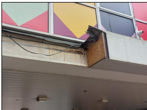
Figure 3: Building 10 showing evidence of deterioration
