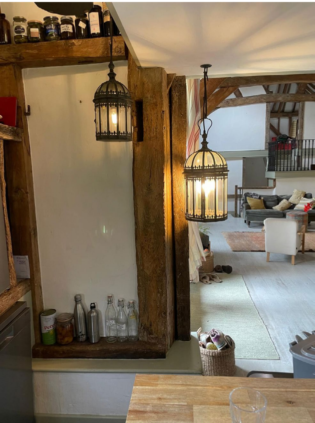
PHOTO D The modern timber fixed in front of the existing post. The modern timber is to be removed.
