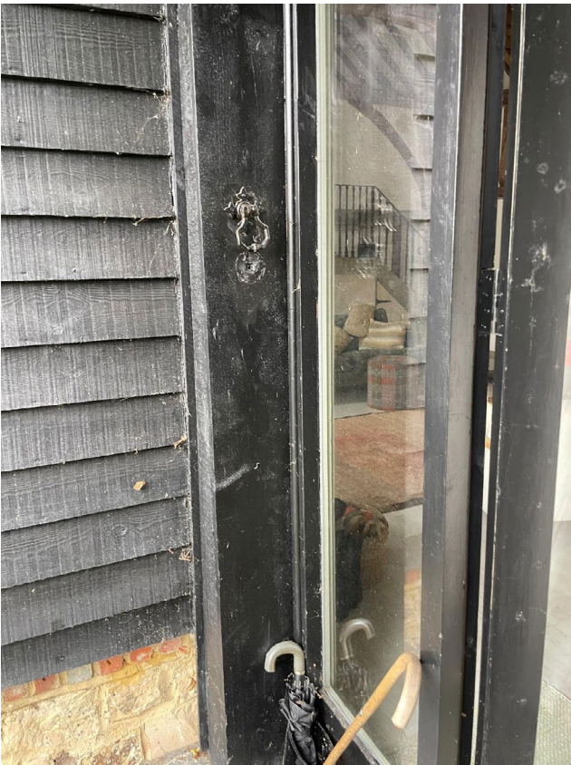
PHOTO B The side of the timber post is not visible
