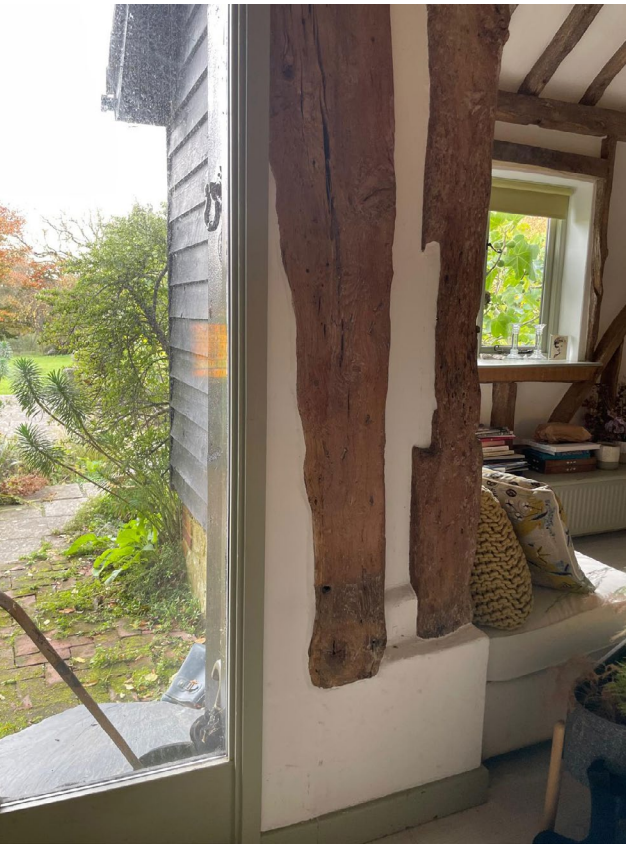
PHOTO A Existing condition shows plaster on side adjacent to door
