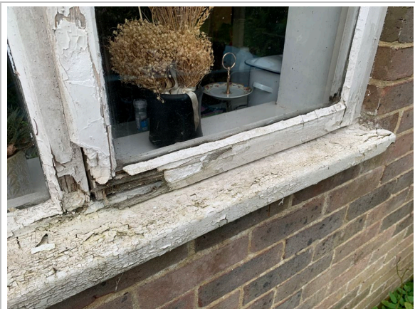
Image of rotten window to the side extension
