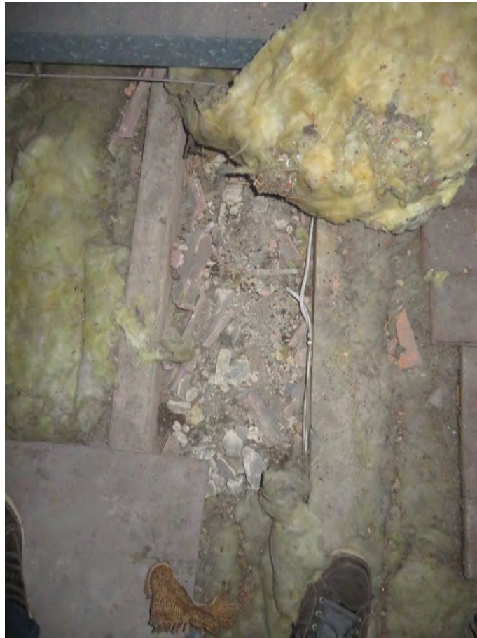
Photograph 11: Debris on ceiling backings
