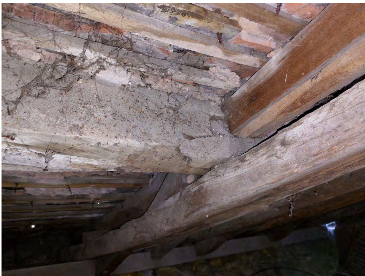
Photograph 4: Fracture to purlin to west elevation of Bay 5
