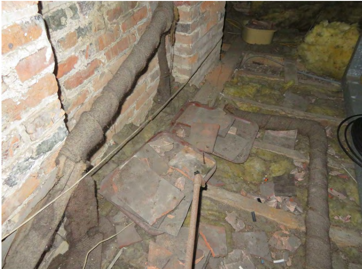
Photograph 12: Debris on ceiling backings
