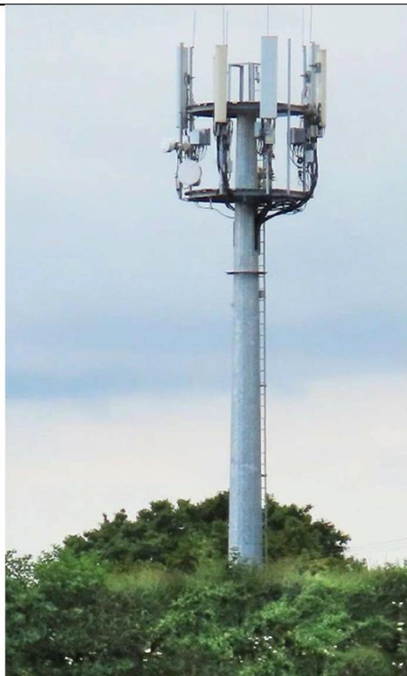
Image 2: Example of monopole with headframe (Source: FLI)
