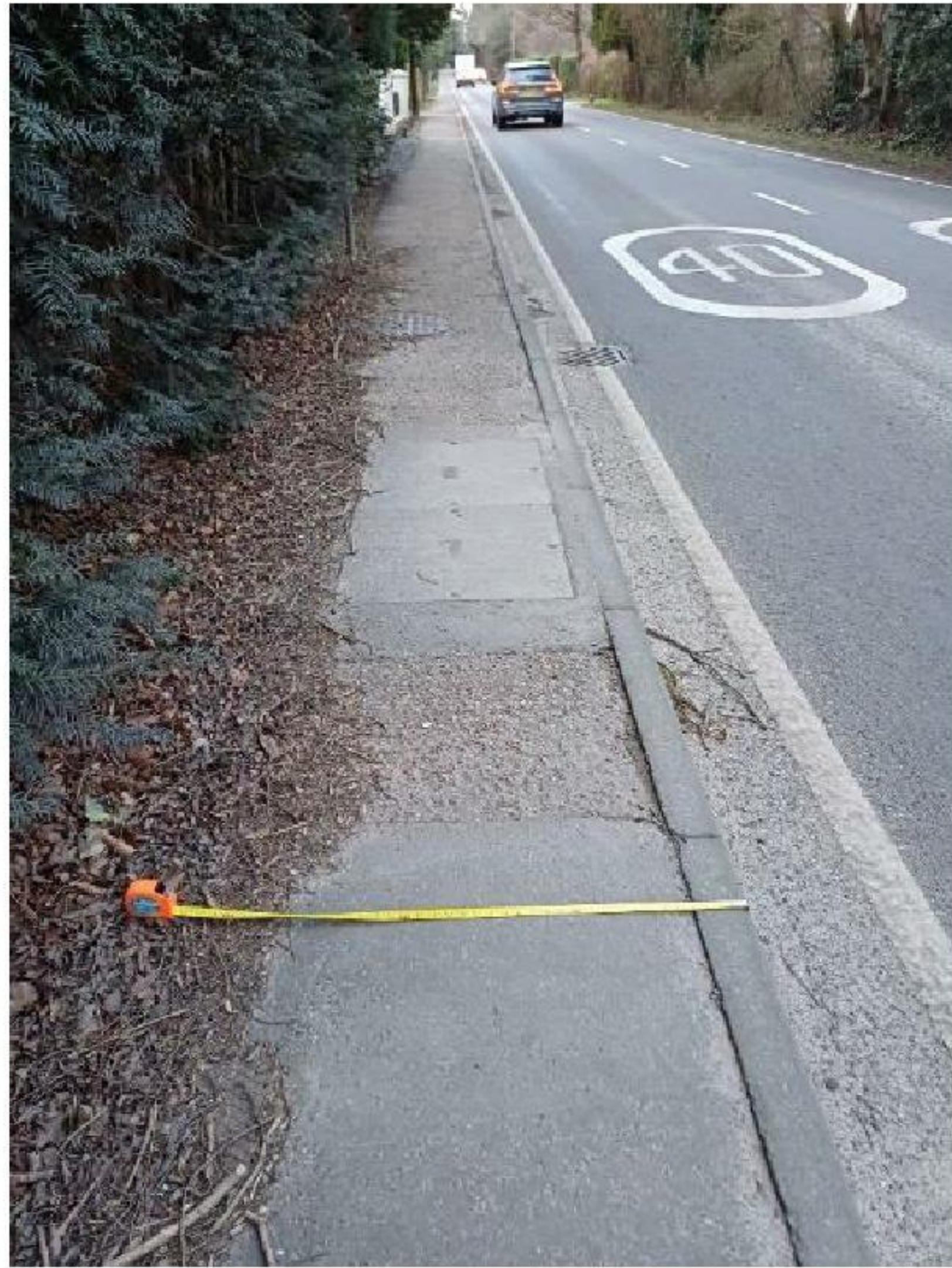
Figure 8 – Lewes Road pavement 10m down from proposed site entrance (tape measure is set on 1m)
