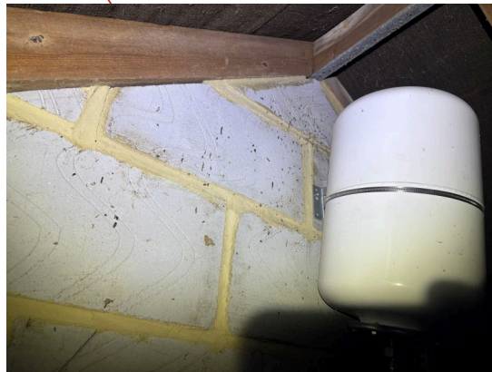
Photograph 2. Approximately 20 bat droppings recorded on the gable end wall within the roof void of the property.
