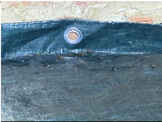
Photograph 2. Approximately 30 fresh brown long-eared bat droppings scattered on the tell tale next to the chimney stack.
