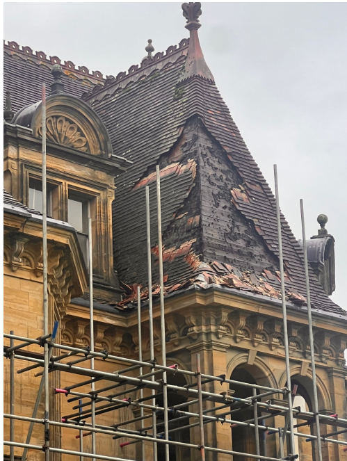
Damaged roof prior to repair
