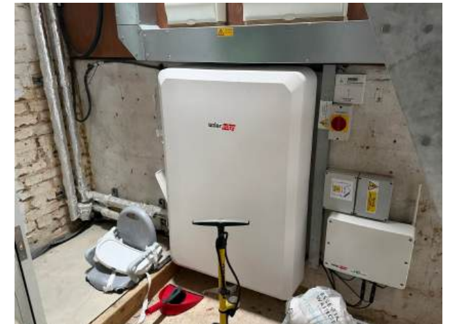
Plate 14 View of battery storage pack in room feature no fabric of interest and other plant equipment.
