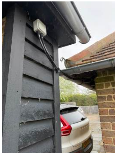
Plate 12 Electricity cable run from workshop to ancillary structure.
