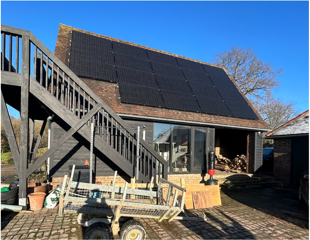
(Fig 02. Photos above, of the workshop with PV's installed)
