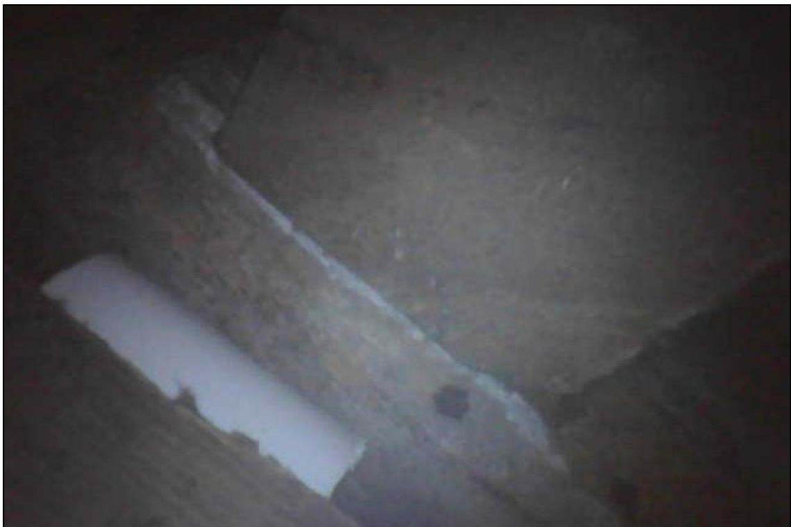
Appendix 2.14: Detail from inspection camera of timber beam above columns in Room 0-09 , (Observation 6) looking north
