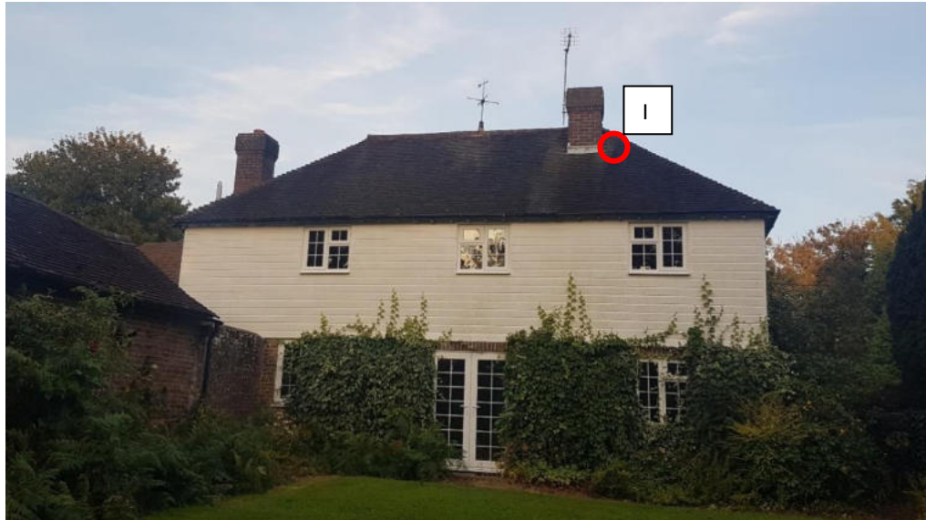
Image 5 – The emergence point of 2 x common pipistrelle from a roof tile next to the chimney on the western elevation of Building B2
