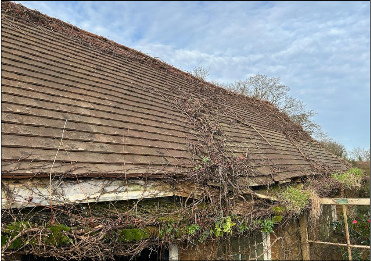
Photograph 1. The eastern face of the potting shed roof, with generally tight-fitting roof tiles, but clear signs of decay.
