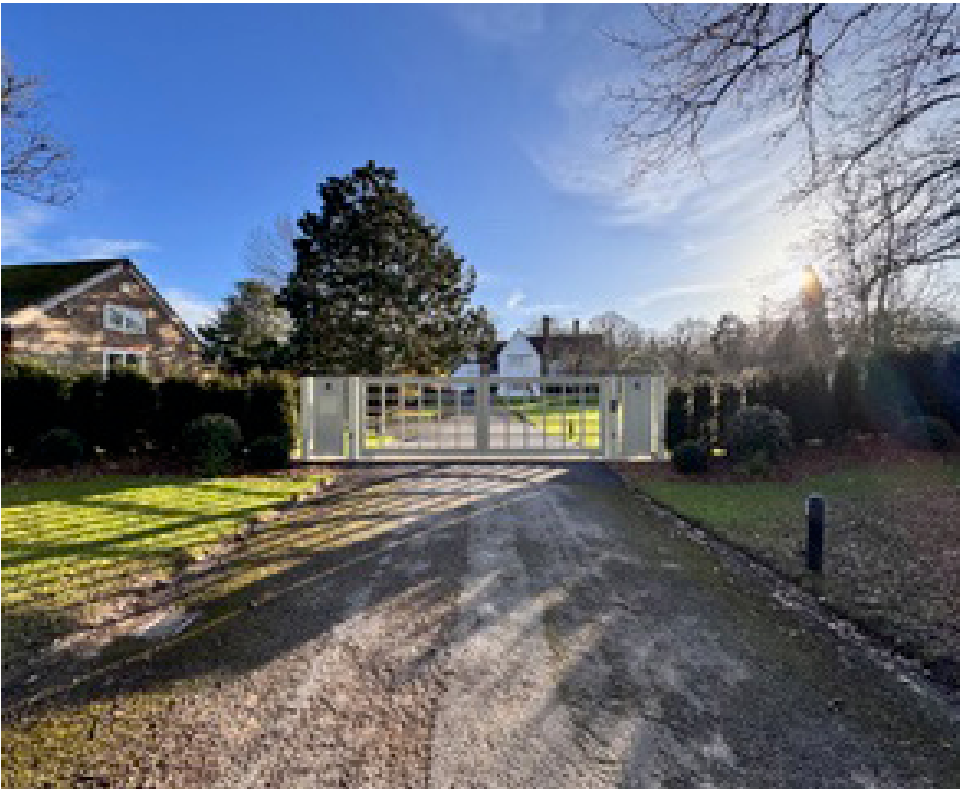
Gate 3 as installed, viewed from the north
