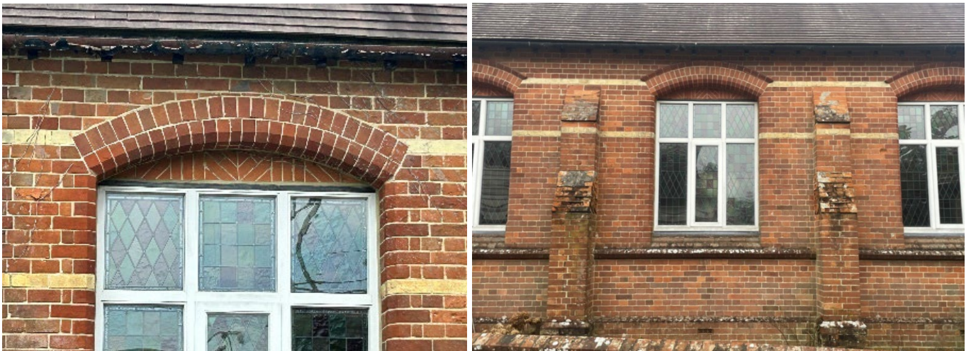
Figure 15: Replacement modern windows to main hall and window head, erroded side buttresses.
