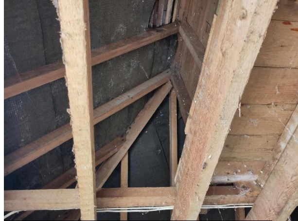
Photograph 6. Internal space of Hurstmead, space open to the felt lining with excessive light ingress from dormer windows.
