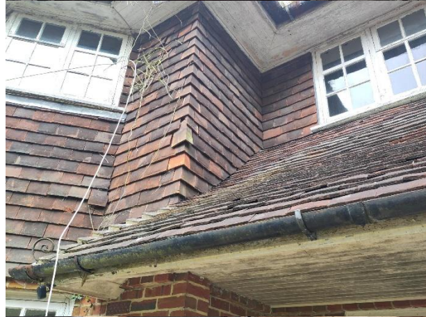
Photograph 5. Loose hanging tiles on southern elevation of property.
