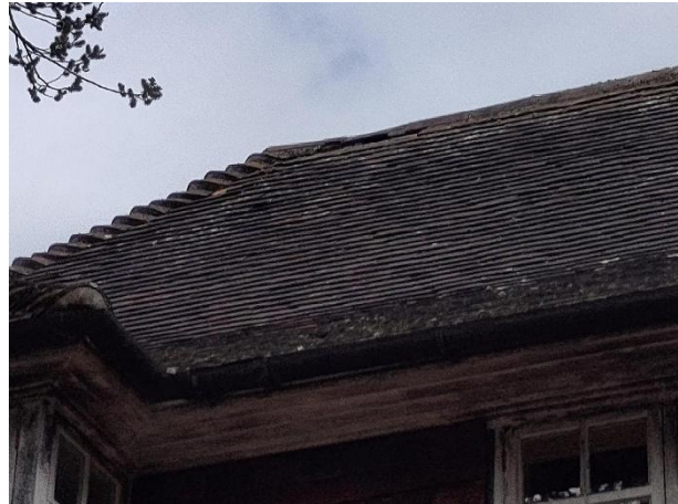
Photograph 4. Gap under ridge tile providing access to cavity.
