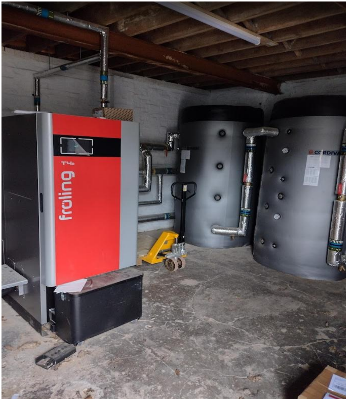
Plant Room Comprising Biomass Boiler and Hot Water Cylinders.
