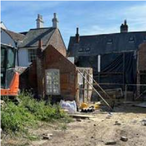
Bake house falling down during strip-out. Photograph provided by the Applicant.
