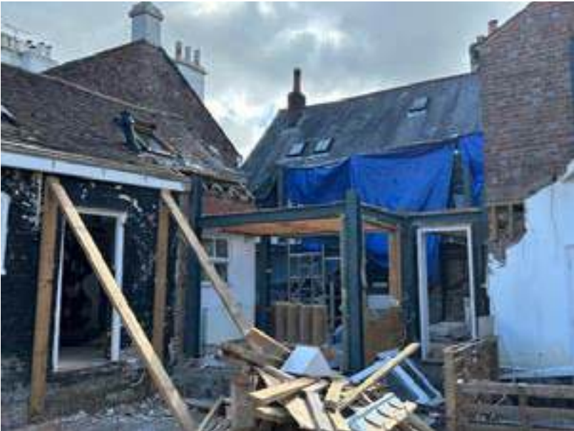
Bake house falling down during strip-out. Photograph provided by the Applicant.
