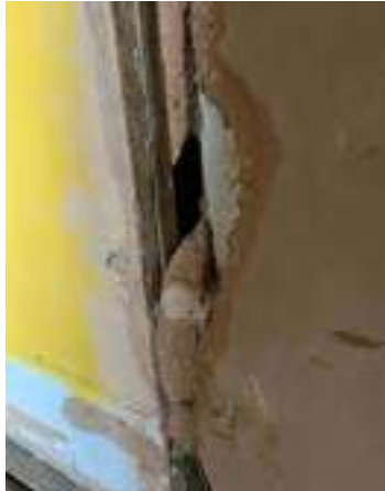
Poor quality bathroom wall before demolition
