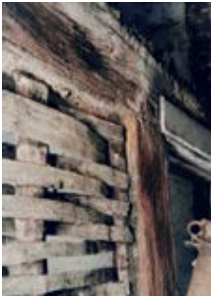
Visible rot and damage observed in the structural support joists within the basement pre construction.
