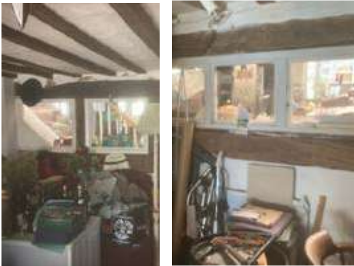
Pre-construction photograph of low quality casement windows, west facade (ground floor)
