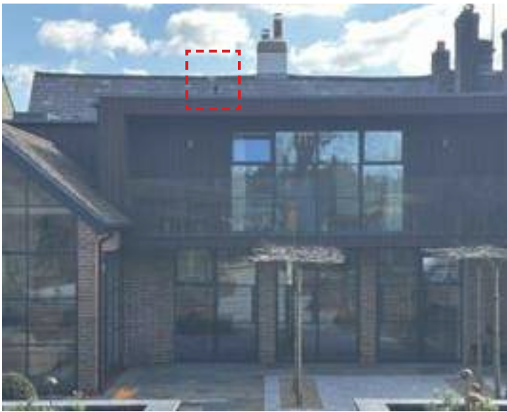
Recent photograph capturing the new boiler flue
