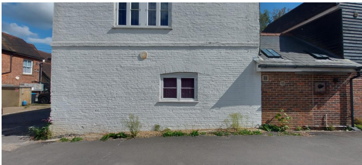
Plate 2. Altered west side ground floor window.
