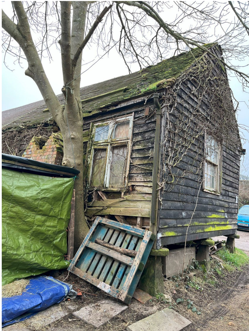
Figure. 13: Rear, south elevation of granary with Victorian or Edwardian four pane casement window and external chimney breast and tree. Rotting timber window frame and cladding evident. (January 2025)
