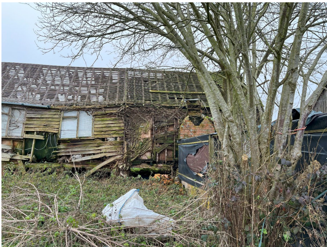
Figure 16: View of south elevation of building 5 showing remnant of brick chimney stack, no roof tiles and significant loss of timber cladding on this elevation (January 2025)
