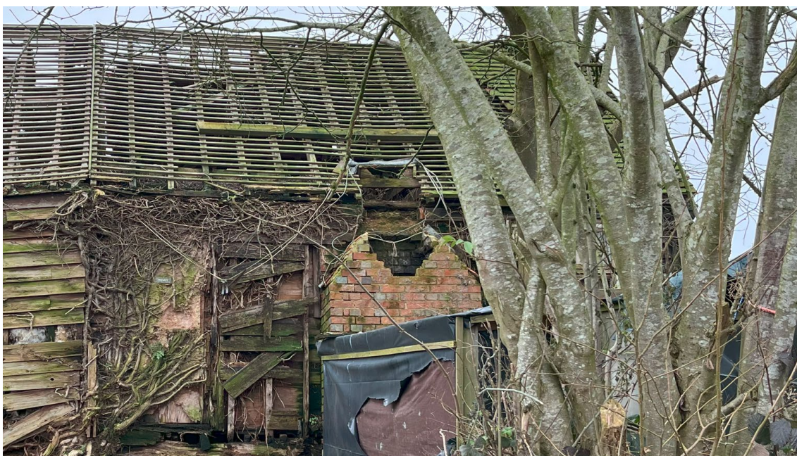
Figure 17: Enlarged portion of Figure 16 showing boarded up rear door, invading ivy plant and layers of chipboard to the left hand side (closer access was not possible. (January 2025)
