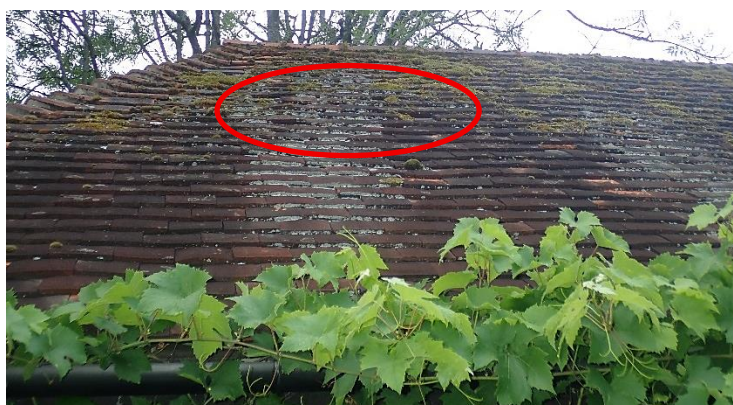
Fig. 6 – Small number of gaps beneath roof tiles, E side of roof
