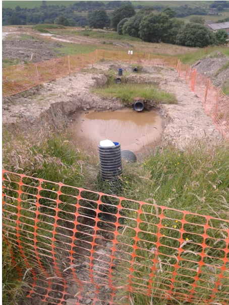
Figure 2: Settlement lagoon and flocculent station
