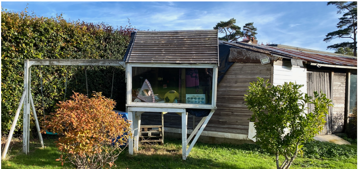
The plastic sheeted and temporary secured roof to part of the gym can be seen here behind the other kids playhouse and swingset.
