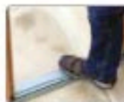
Low level door threshold
