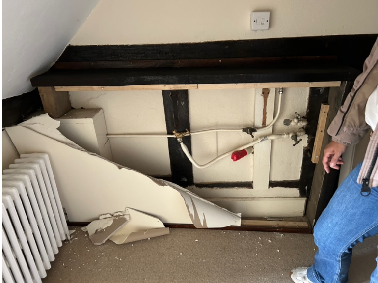
Figure 1 modern plasterboard to boxing in to 2 nd floor bedroom revealing previous pipework
