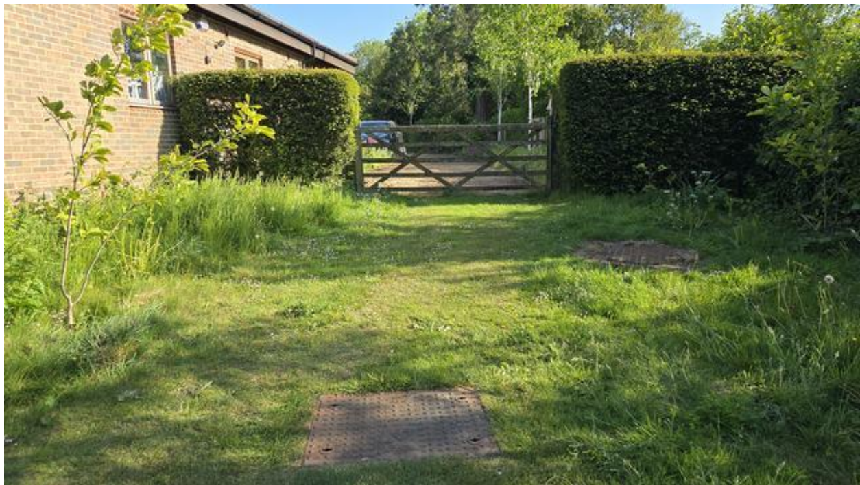
Image 8 Area of proposed garage with a cover over the pumping station that is moving.
