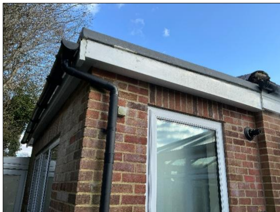
Photograph 3. Gap between uPVC fascia and brickwork on north-western elevation
