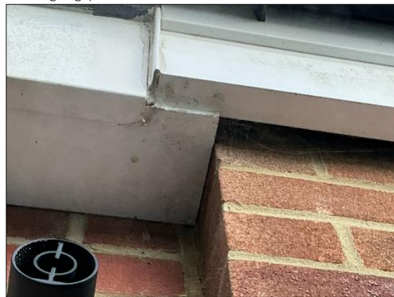
Photograph 4. Heavily cobwebbed gap under fascia in same location
