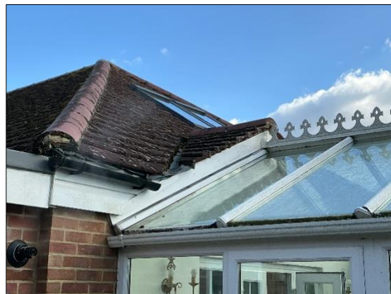
Photograph 2. North-western elevation of main property with slight gaps under roof tiles
