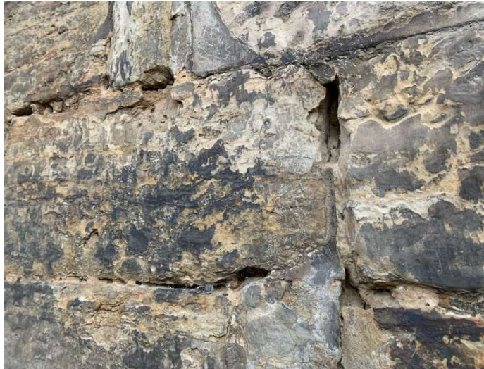
Figure 7-26 – Example of Missing Grout
