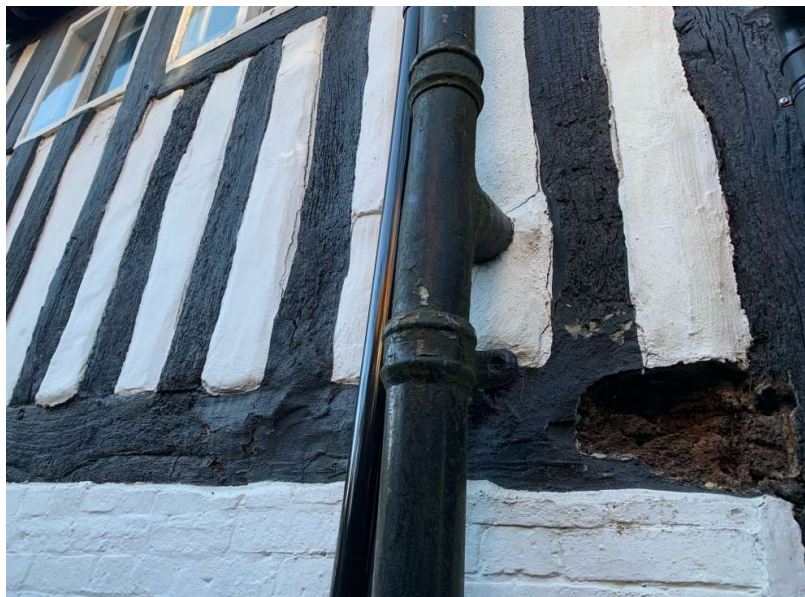
Figure 7-14 – General Area of Damage
