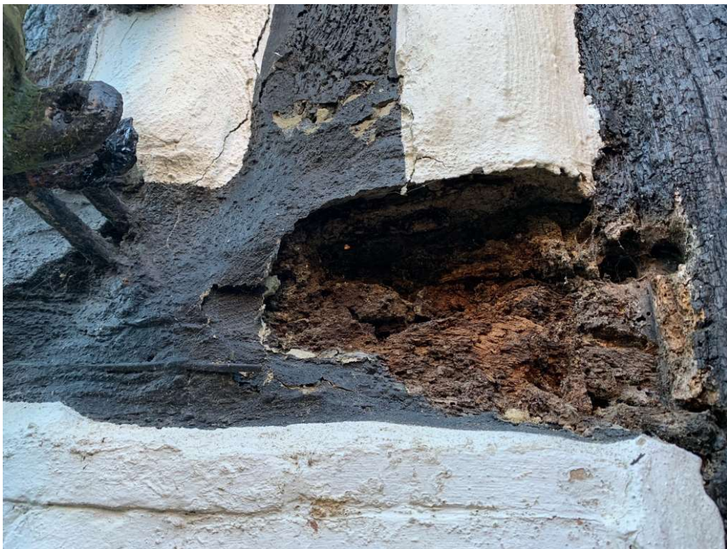
Figure 7-16 – Damage to Timber
