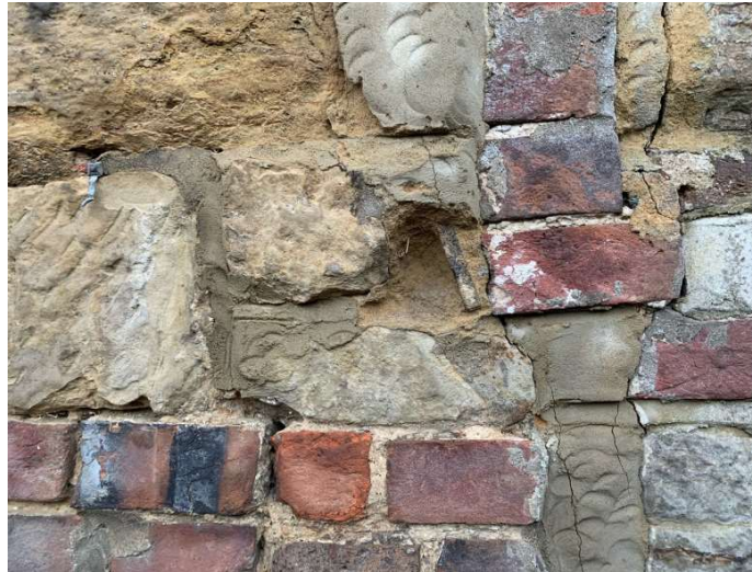
Figure 7-25 – Example of incorrect materials - External
