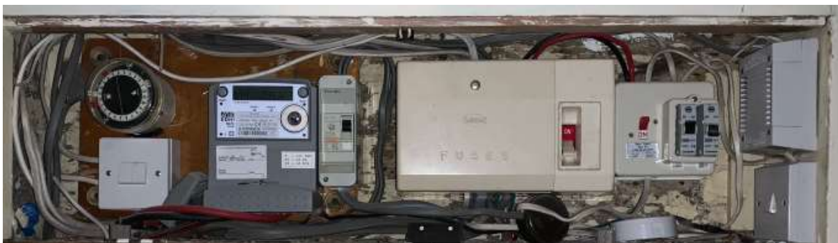
Figure 7-63 – Existing Consumer Unit
