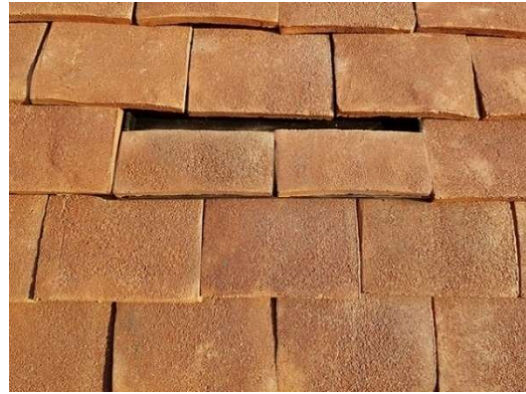
Figure 7-62 – Installed Vent Tile Example
