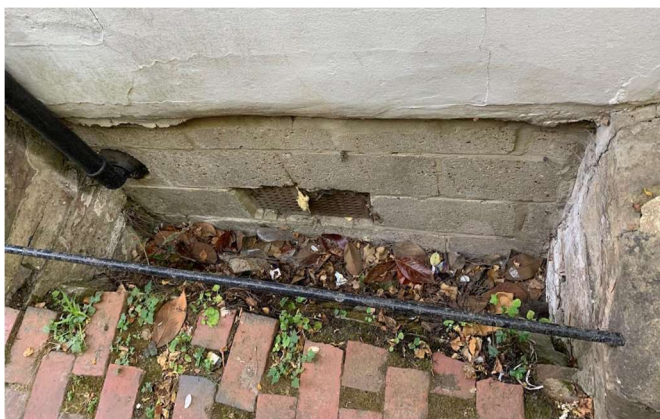
Figure 7-17 – Blocked up Window
