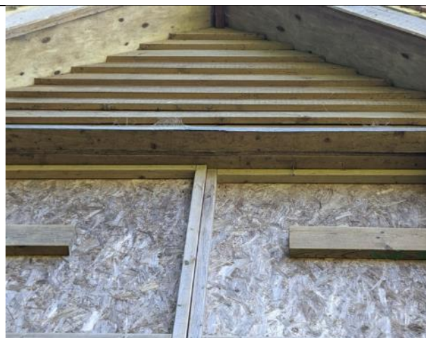
Photograph 6: Gaps in the weatherboarding on the eastern gable hayloft door.
