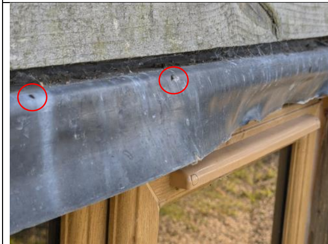
Photograph 3: Small bat droppings below the weatherboarding on the northern gable end.
