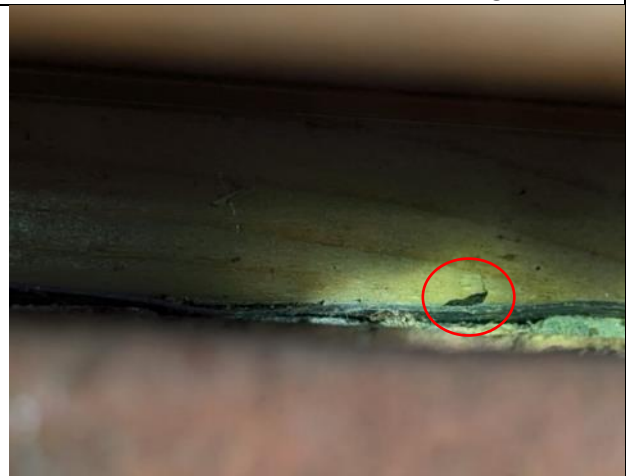
Photograph 4: Small bat droppings in the crevice below the window on the northern gable end.
