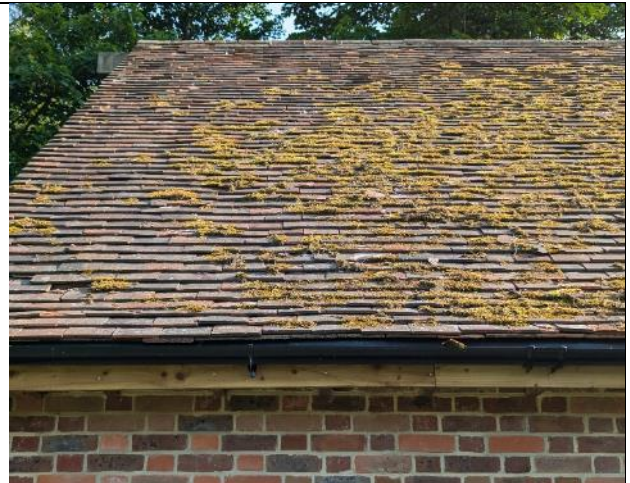
Photograph 2: Missing and lifted tiles on the north elevation of the east wing.
