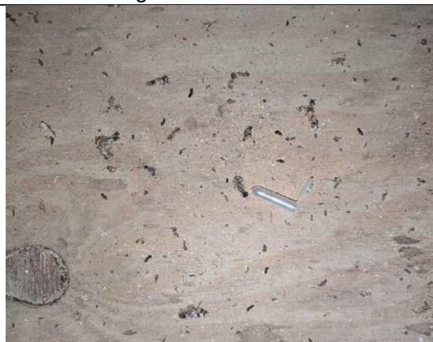
Photograph 10: Small accumulation of medium-sized bat droppings on the temporary boarding at the joist level.
