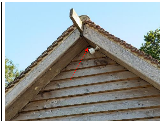
Photograph 5: Gap at apex on the northern gable end.
