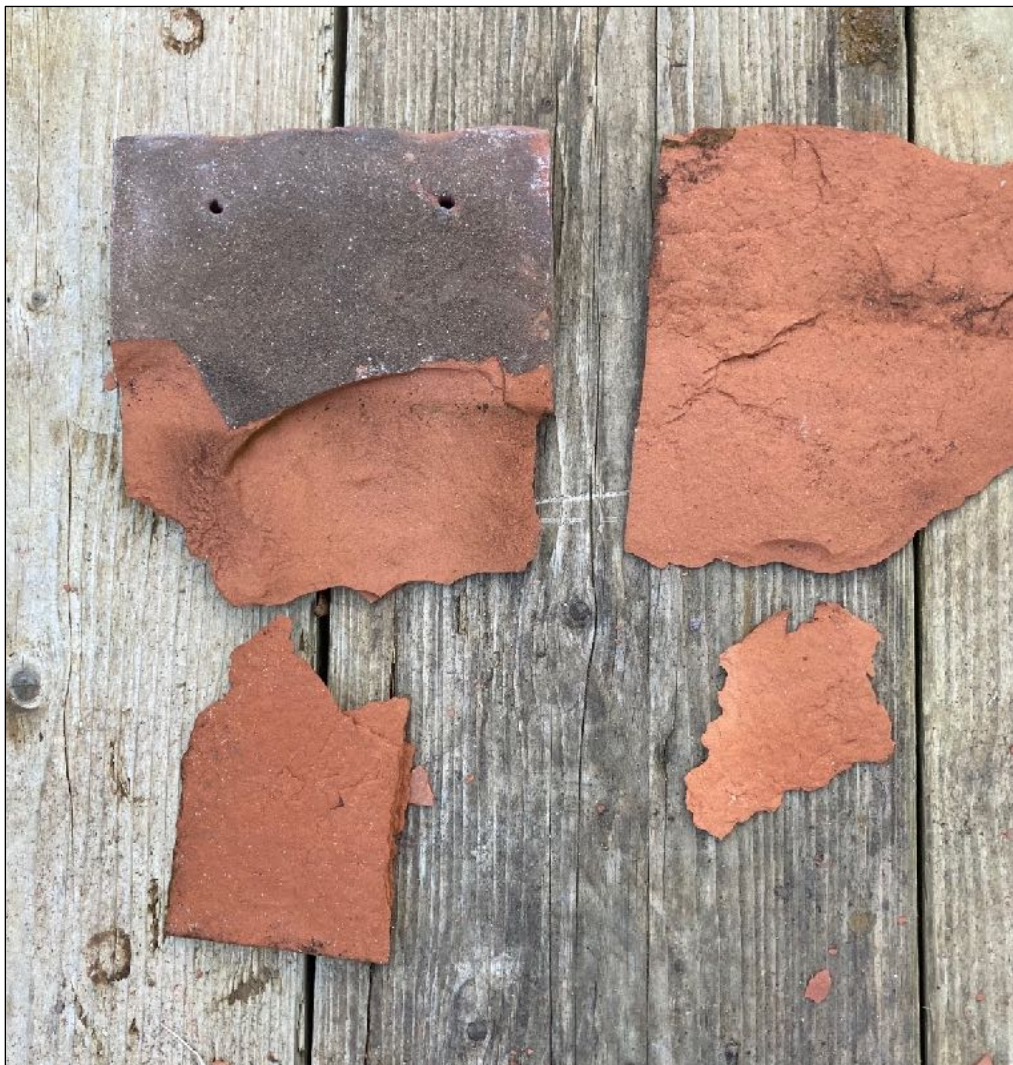
16 – Sahtas tiles, crumbling
