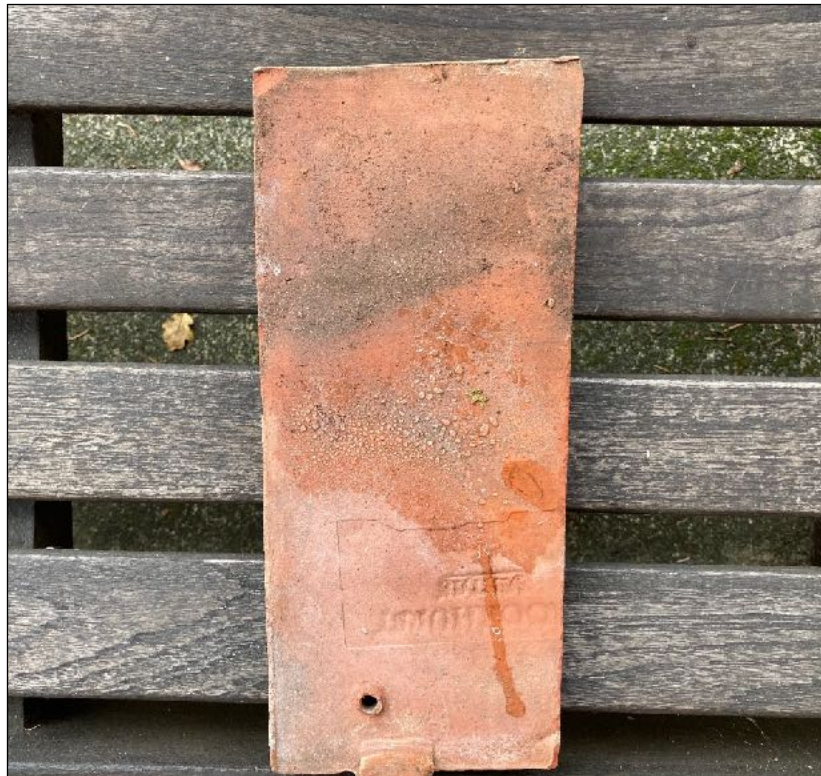
15 – Underside of Sahtas tile when removed, soaked with moisture
