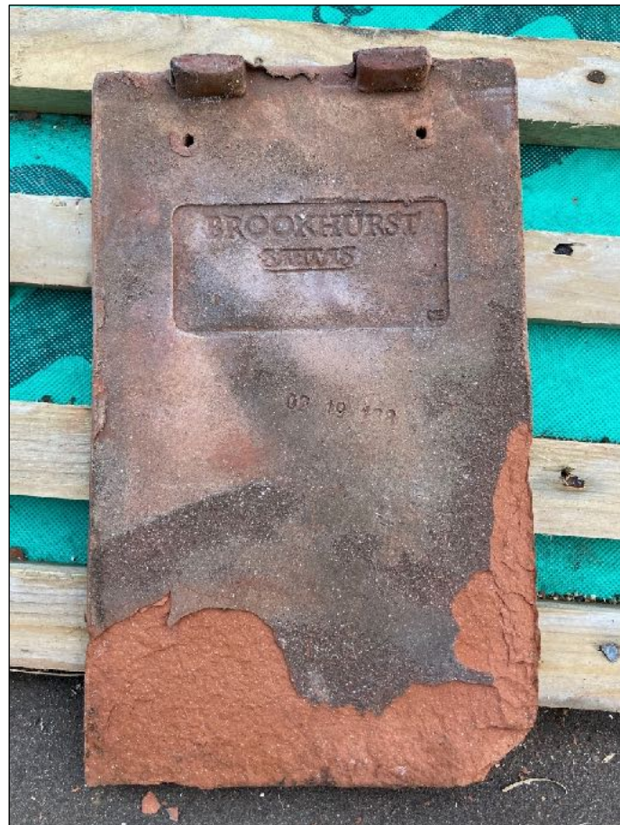
18 – Underside of Sahtas tile delaminating, upper surface intact
