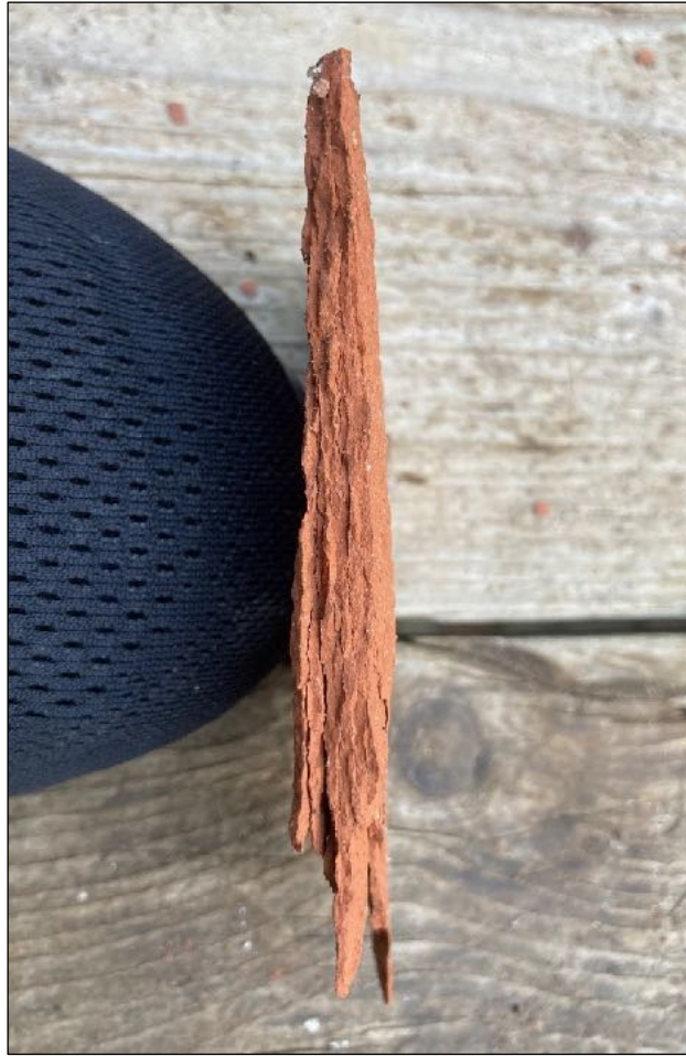
17 – Sahtas tile, showing delamination
